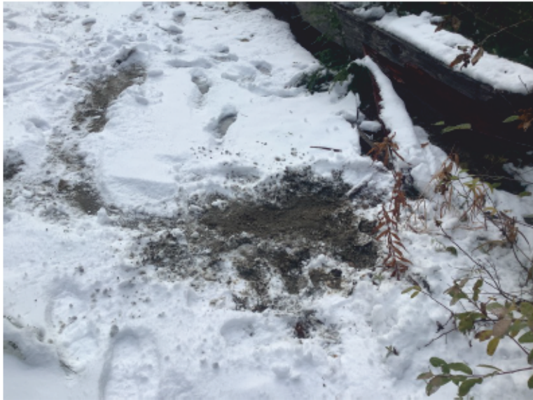
Ballast wall still sitting low of panel. Fix fro, previous inspection not complete
