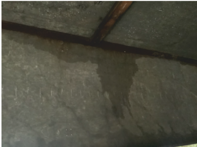
Evidence of leaking joint
